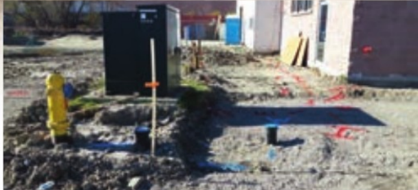
Digging directly on top of locate marks is always an unsafe practice. Even minor inaccuracies or discrepancies in depth data could create a dangerous situation.
