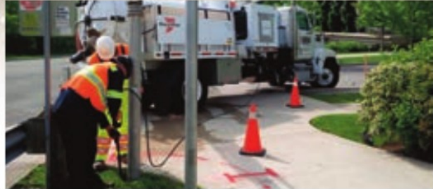
Be sure to limit excavation to the area covered by the locate request submitted to, and processed by, ON1Call.
